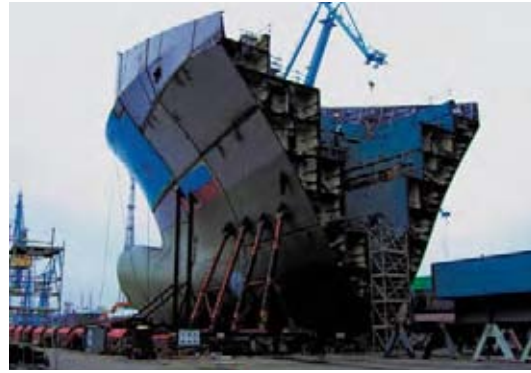
3 Bow section of a fast containership built on keel blocks: In shipbuilding today, the individual sections are pre-fabricated and then assembled to form the ship's body. Thanks to a system of rails, the ship can be moved about the shipyard according to work requirements. Source: Fraunhofer AGP
